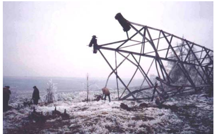
Fig. 7. Foundation failure of OHL 330 kV “LadTES – DsGRES”
