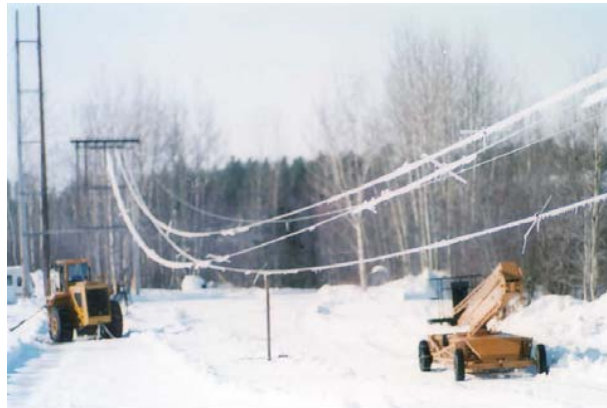
Photo 2 View of partly shed conductors (first event)
