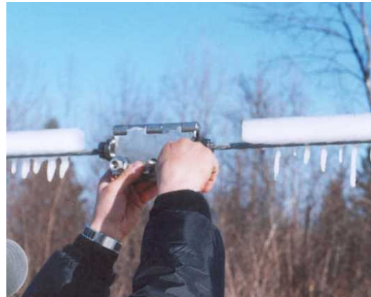
Photo 8 Plates attached by screws to the cable ensuring no damage is caused to the surface.
