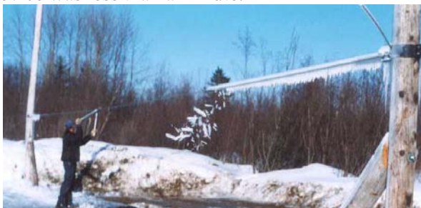
Photo 10 De-icing of the 15 m long cable after a few degrees of twist. °
