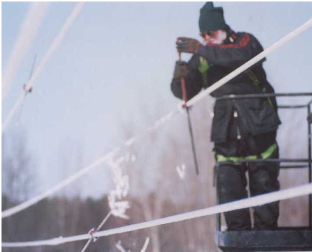
Photo 1 De-icing along few meters at the start of iced cable rotation. (February 2003 de-icing test)
