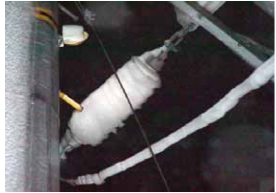
Fig.7 Long rod insulator covered with wet-snow
