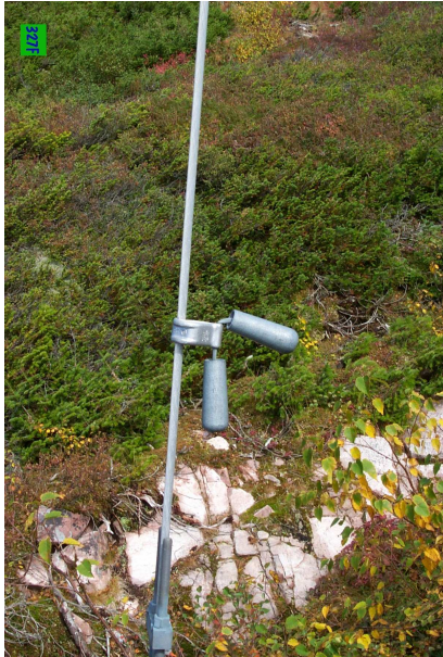
Figure 4: Typical damper failure of initial damping solution for guy support cables
