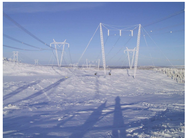
Figure 1: Rime accretion on James Bay network structures
