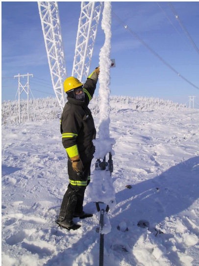
Figure 2: Large hard rime accretion on guy cable
