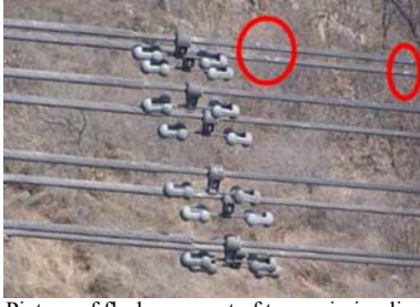
Figure 11. Picture of flashover spot of transmission line of 667th
