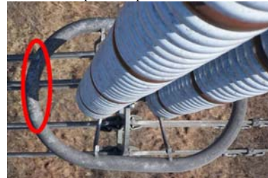
Figure 9. Picture of flashover spot of grading ring of 667th
