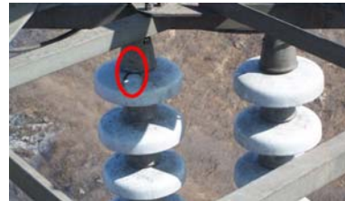
Figure 8. The flashover spot of A phase small side insulator of 667th
