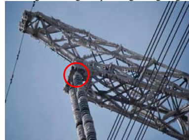
Figure 6. Icing condition of insulator and cross arm of A phase after flashover(front side is small side)
