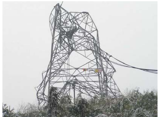
Fig.1: #390 collapsed tower of 500 kV Wumin line
