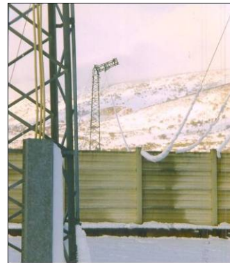
Fig. 1: lattice tower fell down, due to overload ice on conductors (Puglia; 1995, Italy).
