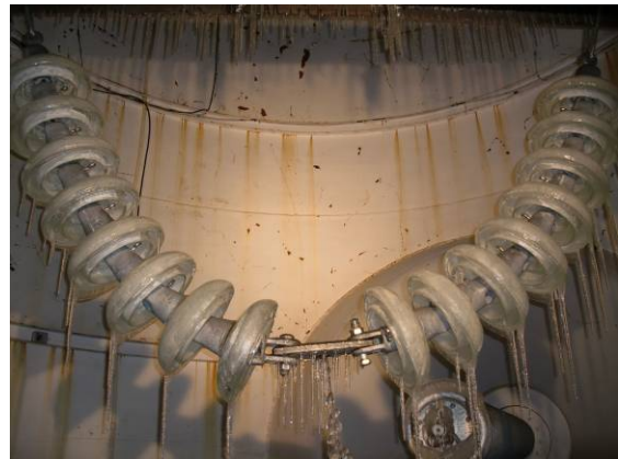
Figure 4. The icing insulators of V-shape suspension strings
