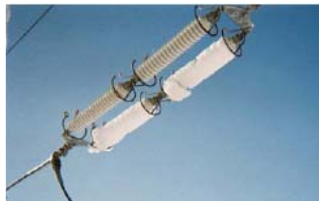
Figure 1. Example of packed snow on horizontally mounted long-rod insulator strings.
