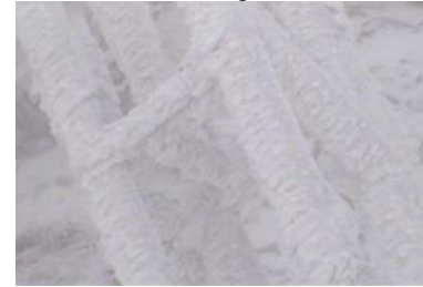
Figure 1. The photo of ice on four bundled-conductor
