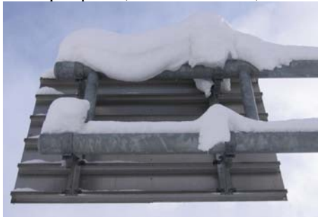
Fig. 1: Snow accretion on road information sign
