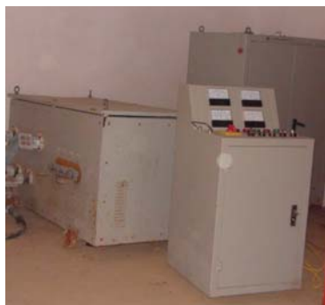
Figure 3. 5000A/800kVA current generator
