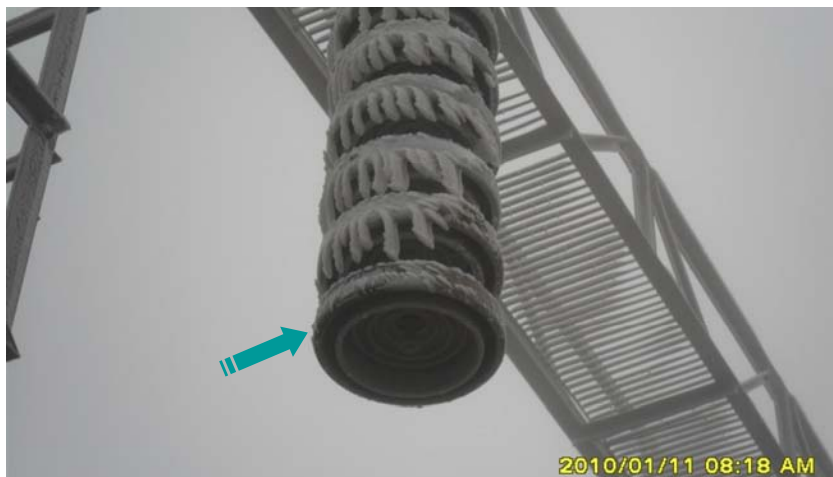
Figure 7 Rime on the insulator string
