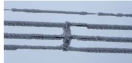
(a) Icing on conductor
