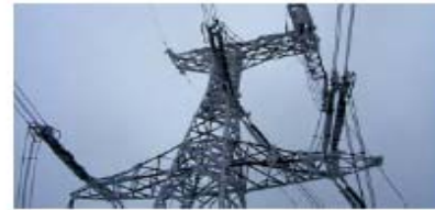
(a) 杆塔覆冰
