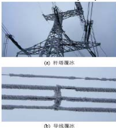
Figure 2: Icing on 109# Tower of Shenyuan I lines
