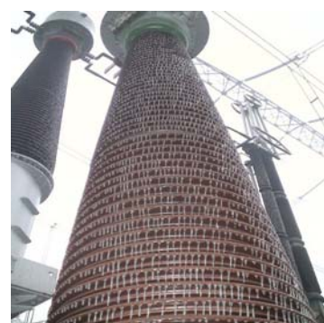
Figure 1: The surface icing state of 5012 Phase B, 500kV YuXian Substation.
