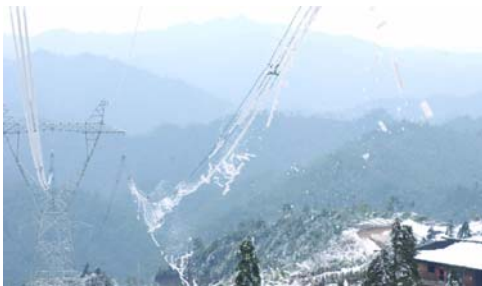
Figure 1. The scene of Ice-shedding of transmission line
