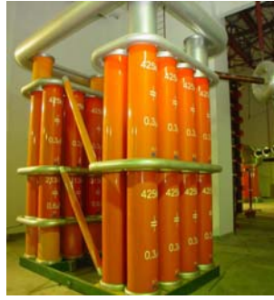
(b) DC \pm 600 kV/0.5A power supply
