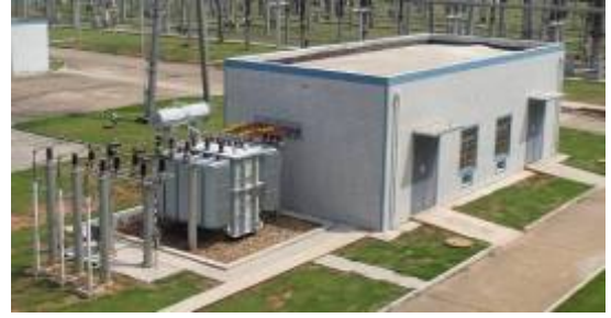
Figure 7: 500kV DC De-icing Device Field
