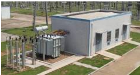
Figure 1: 500kV DC De-icing Device Field
